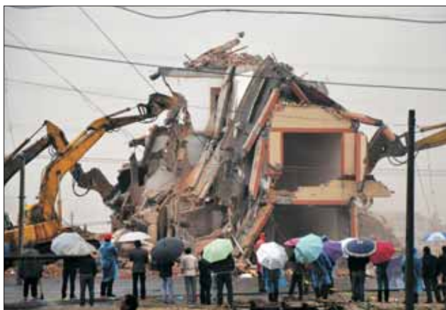
HOLDOUT SELLS. A house in the middle of a new road is torn down on the outskirts of Wenling city in eastern China's Zhejiang province. Authorities have demolished the five-story home that stood incongruously in the middle of the new main road and had become the latest symbol of resistance by Chinese homeowners against officials accused of offering unfair compensation. (AP Photo)
